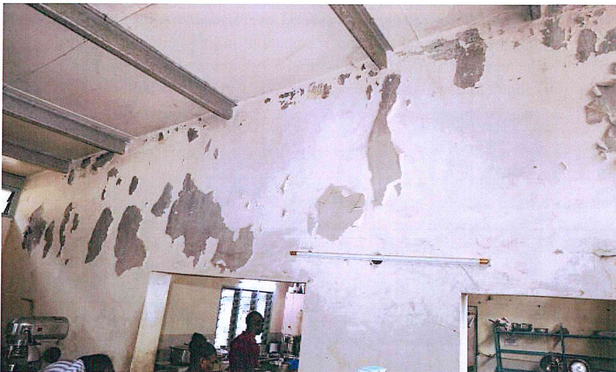
Picture 4: The Committee observed widespread infrastructural deterioration with worn-out floors, walls and peeling paints witnessed in majority of the hospital wards visited.
