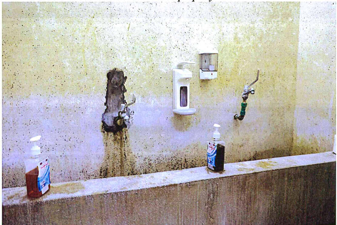
Picture 7: There was widespread deterioration and wearing out of the facilities at the wards especially in the bathrooms
