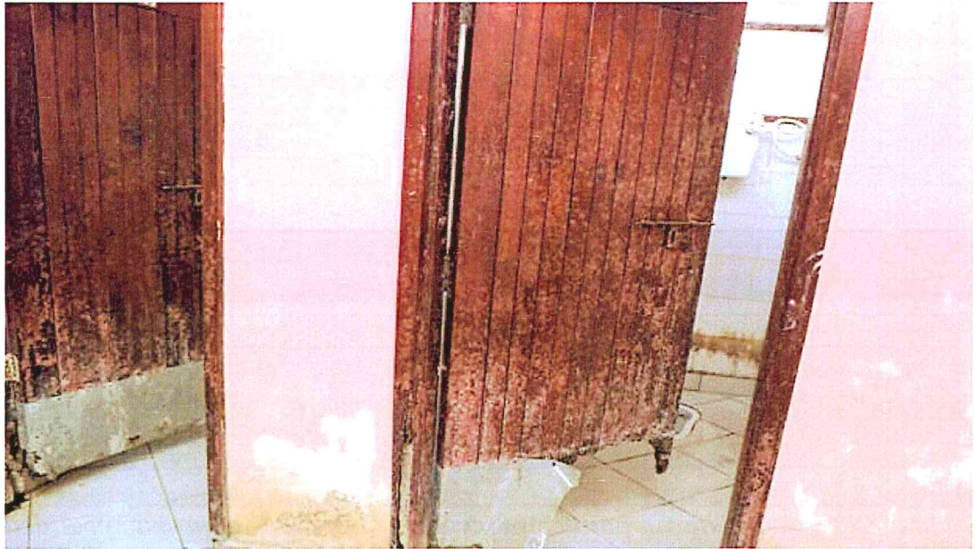
Picture 6: The bathroom doors were missing and where present they were worn out and unable to lock properly.
