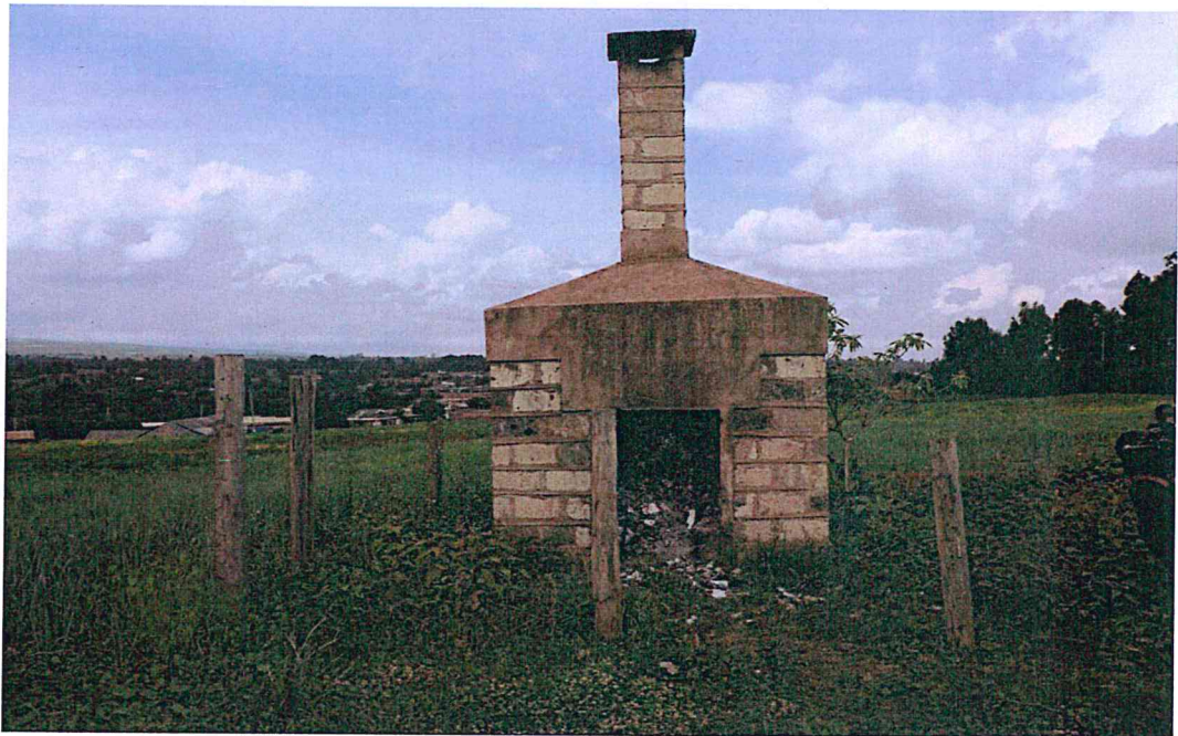
Picture 13: The committee observed that the hospital incinerator lacked a functional door and perimeter fencing, raising significant concerns regarding environmental safety.
