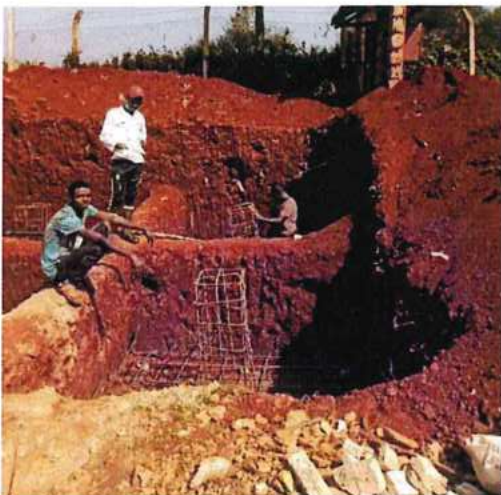
Construction of reinforcement cages and stub Columns for the Water Storage tank at KNH Othaya
