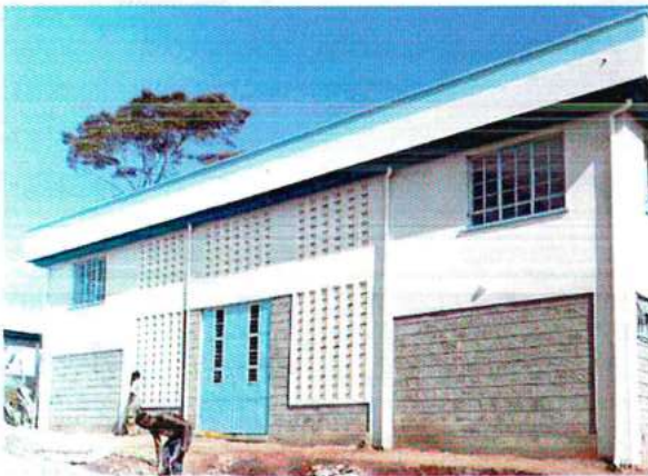
Construction of the KNH-Othaya Oxygen Plants
