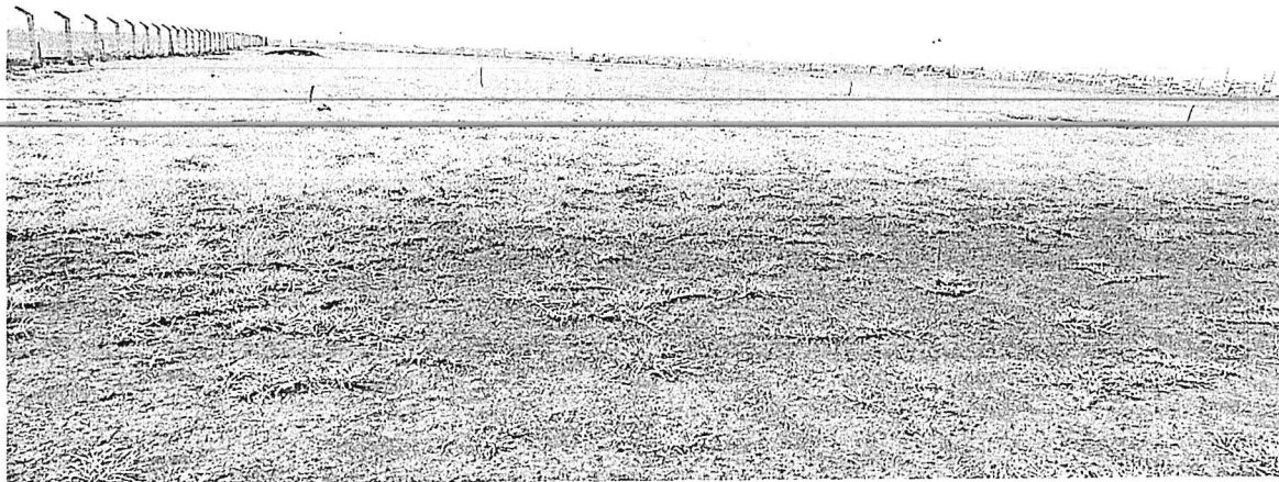
Fig 20: levelling and replanting of grass is complete for Rugby pitch and Football pitch 2. Football pitch 1 is 90 % complete.
